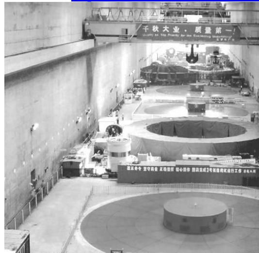
THREE GORGES DAM – TURBINE HALL
